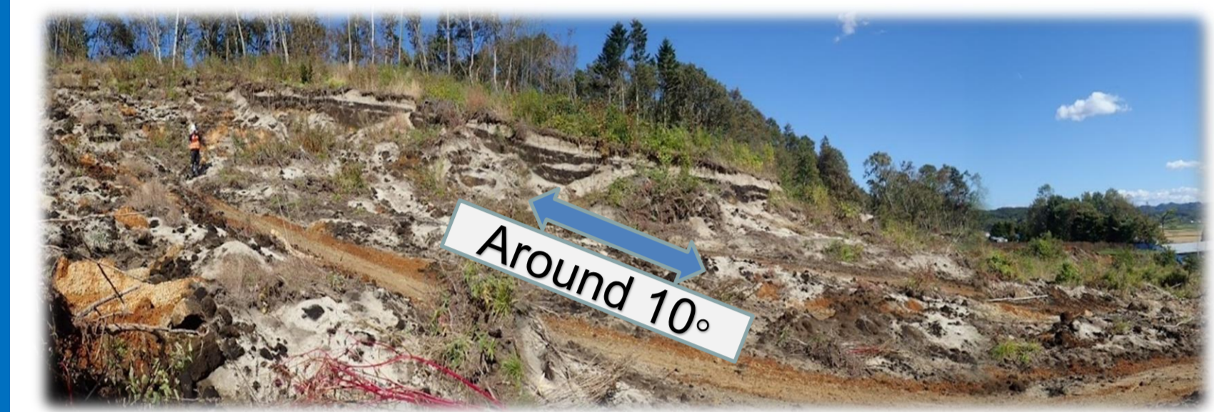
Slope failure after 2018 Hokkaido Eastern Iburi Earthquake
