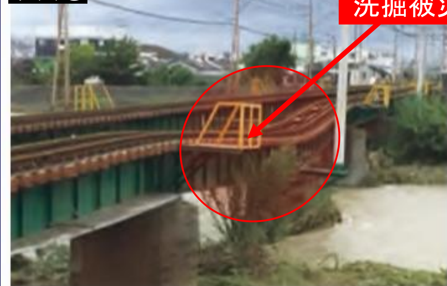
洗掘被災の事例
